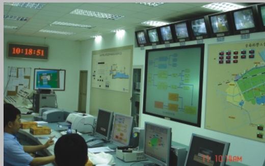
24-hour Monitoring on Dajhou Water Level and Rainfall at the Flood Control Center
