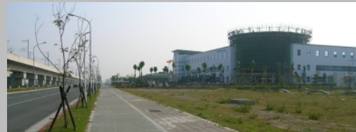
The Site after Completion of the Elastic Vibration Reduction Wall Construction (The Wall was Built on the Strata Under the Right Side of the Pavement. The Ground Restoration was Completed.)
